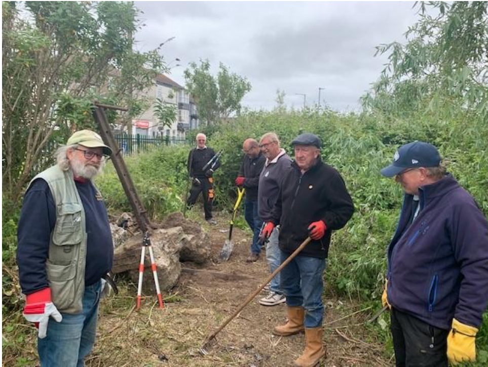
Picture of the Shed Members clearing the ground for their new Shed beside the railway tracks at Lowestoft
